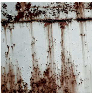
Protection from rust and corrosion
